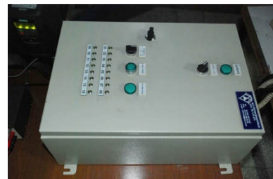
Figure A.12: Valves control unit.
