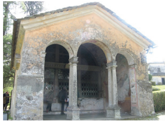
Fig. 4 Decay of historical plasters because of the rain infiltrations (Chapel n. 13—The Temptations).
