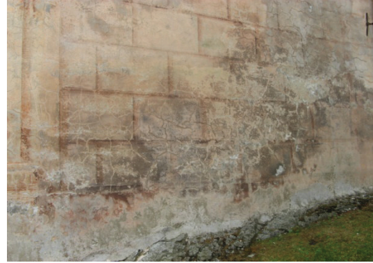
Fig. 3 Delamination and detachment of artistic plasters because of the rising damp effects due to capillary action or rain infiltration (Chapel n. 23—Jesus is taken).
