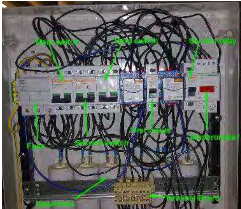
Figure 22 Image of the control board
