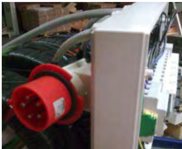
Figure 23 Image of the power point wich powers the control panel
