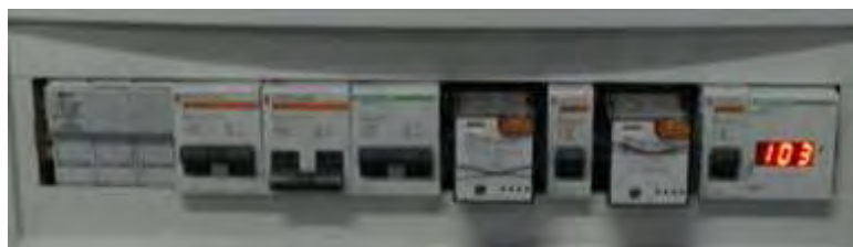
Figure 24 Image of the control panel
