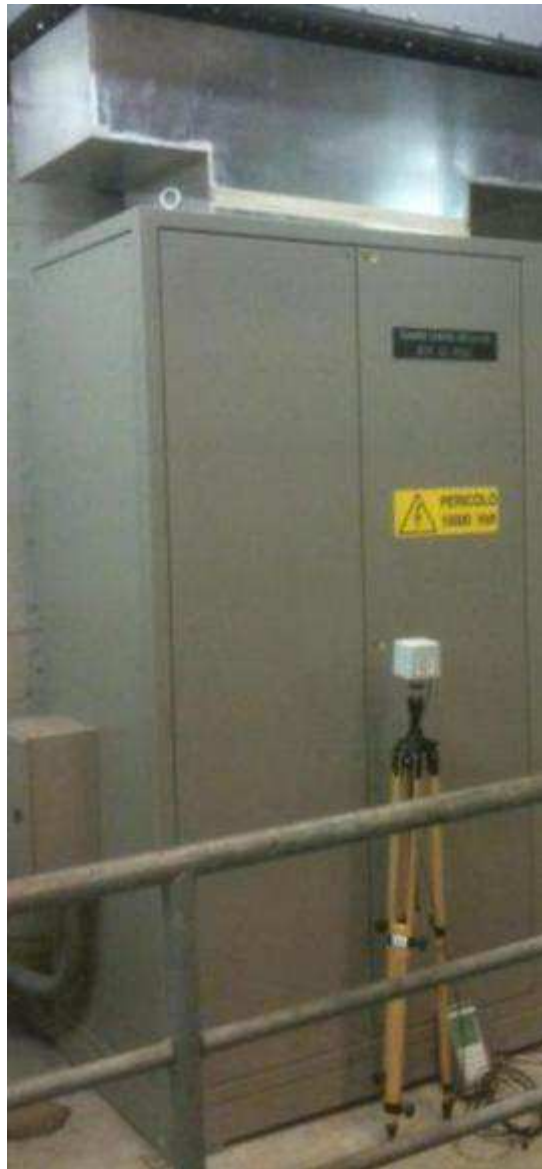
Figure 39 Image of the electrical cabinet
