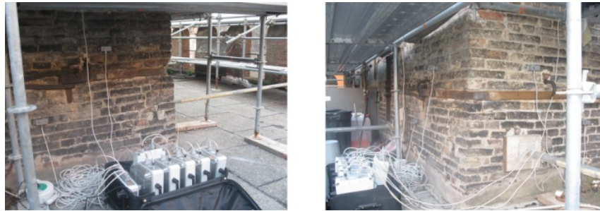
Figure 4. Photos of the AE data acquisition system on the monitoring site.
