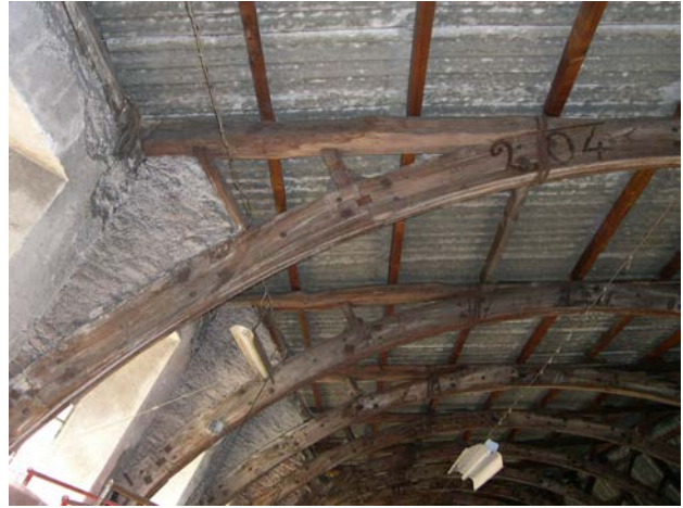
Figure 8 – The former Gallo wool mill, Sagliano Micca (Biella). Detail of the assembly system of the boards. (photo Mattone).
