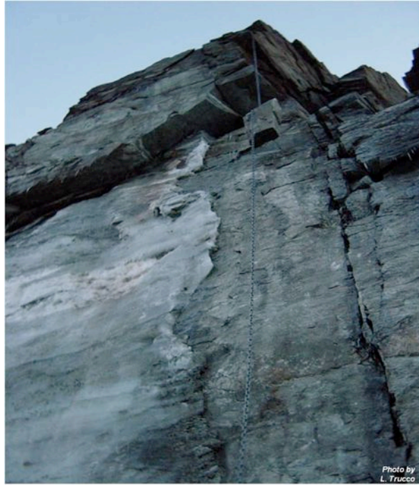
Figure 3.1: The ice lens (of about 15 m high and 7 m large) observed on the detachment surface after the “Cheminée” rockfall occurred on August 18th, 2003 (Photo by L. Trucco).
