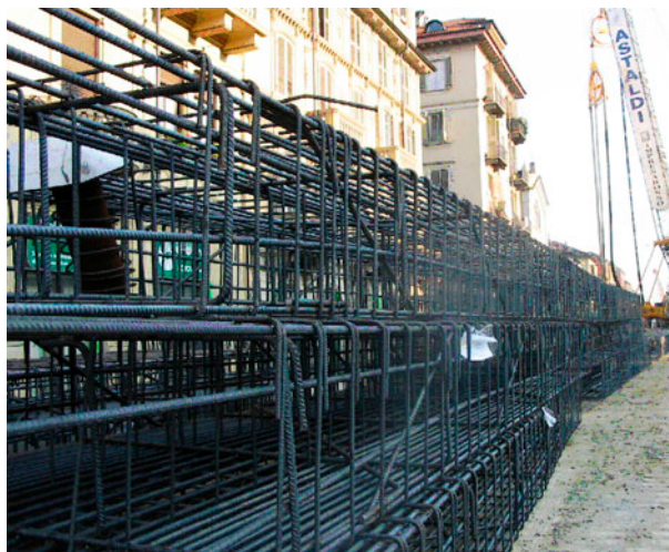
Figure 2. Diaphragm reinforcements in the site area of the Turin railway link ready for insertion into the panels excavated by means of trench-cutters.
