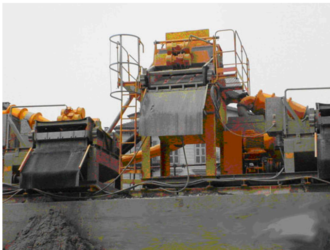
Figure 5. General view of the desanding system of the bentonite mud used for the Turin underground railway link.
