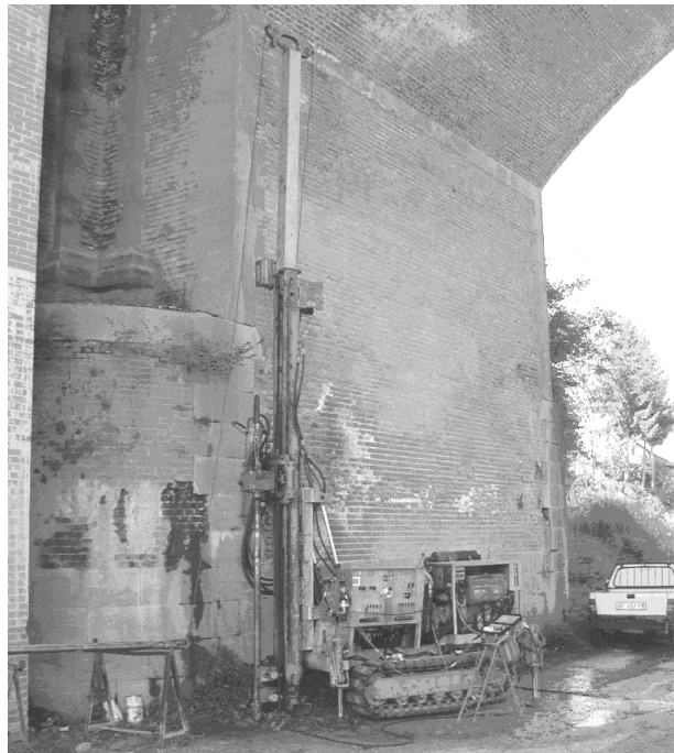
Fig. 3. Drilling equipment used for the core destruction monitoring drilling on the shoulder of the bridge over the Gesso Stream at Cuneo
