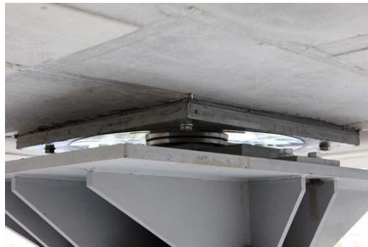
Figure 29: A single pendulum bearing in situ. In this installation the sliding surface is faced down.
