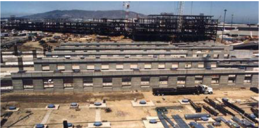
Figure 33: The arrangement of the Friction Pendulum during the construction phases of San Francisco's International Airport, www.earthquakeprotection.com .
