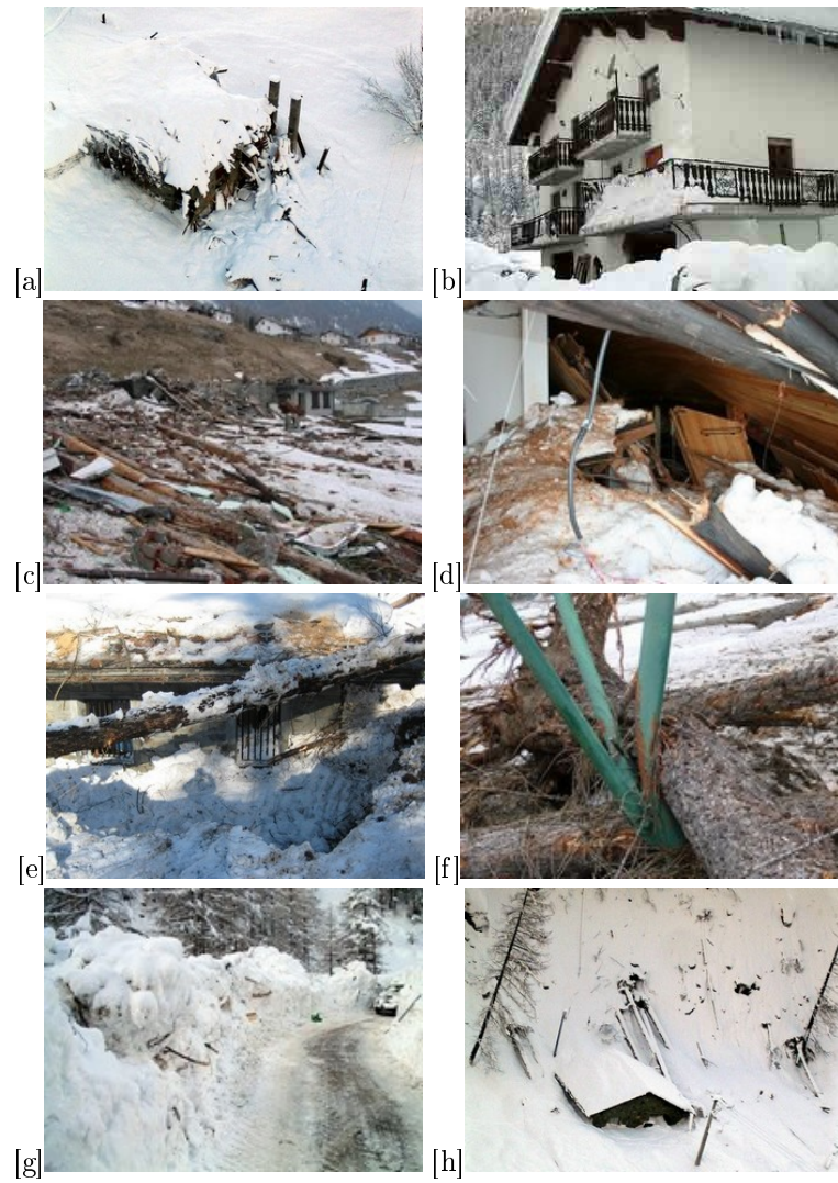
Figure 6.4: [a] House n. 3 destroyed. [b]-[e] Houses damaged. [f] High voltage pylon damaged. [g] Deposit on the road. [h] Trees crushed. Photos RAVDA.
