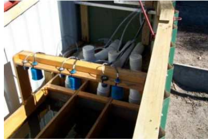
Fig. 36 – Depth sensors for the detection of the outflow discharge
