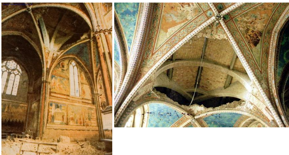
Figure 2.9 - Collapse of the vault of the San Francesco Basilica in Assisi after the 1997 earthquake.
