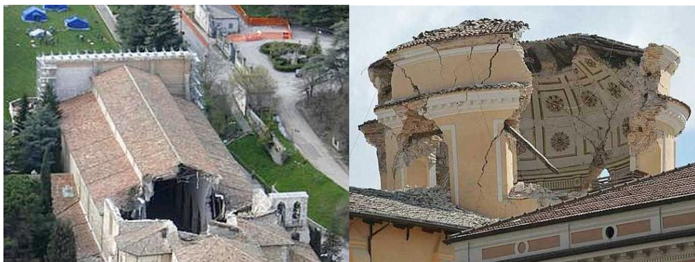
Figure 2.11 - Basilica of Santa Maria di Collemaggio (left-side), Church of Anime Sante (right-side).
