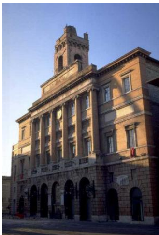
Figure 2.10 - Damage occurred to the Civic Tower of the city hall in Foligno after the 1997 earthquake.
