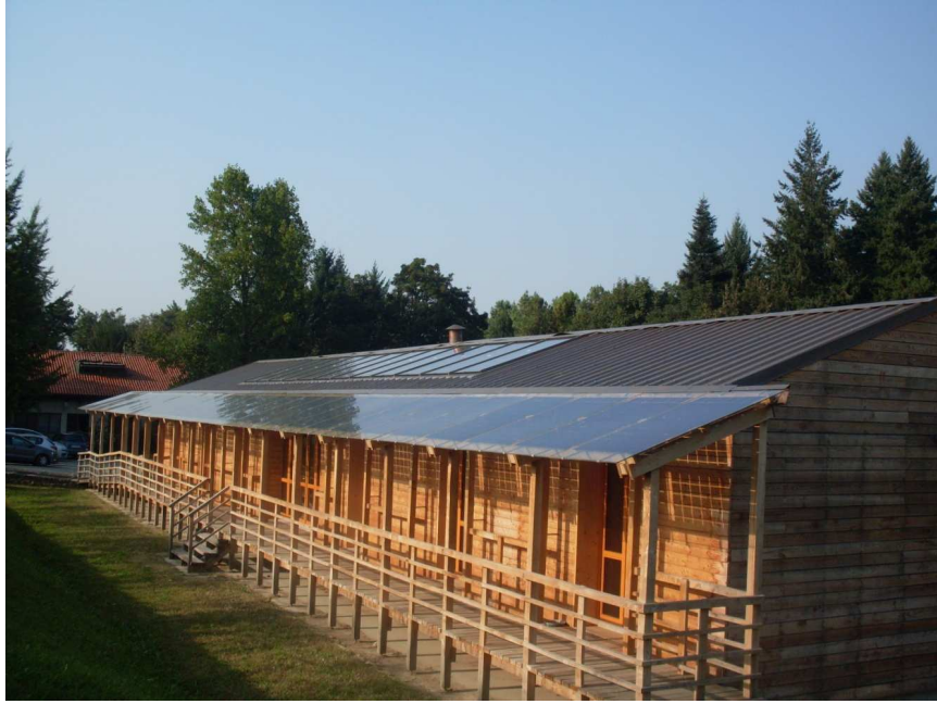
Figure 79 Solar thermal collectors and PV collectors on the roof of PUEEL building
