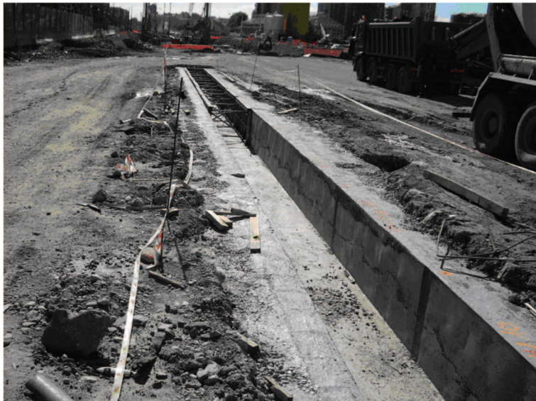
Figure 5. View of the short trench made initially to allow excavation of a panel in order to begin the construction of concrete diaphragm walls.
