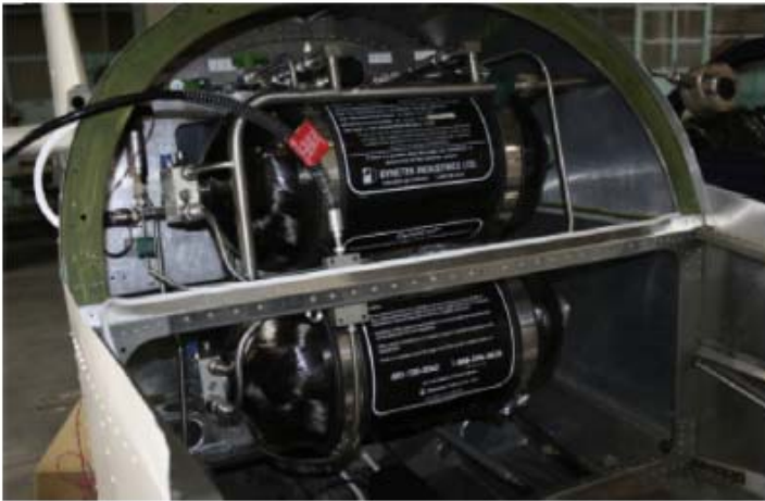
Fig. 5 Hydrogen storage system.
