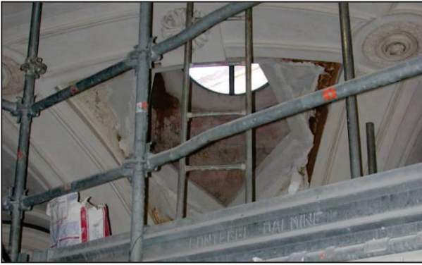
Fig. 5 - Opening of the six pentagons located in the dome above the altar after the untap the paint surface
