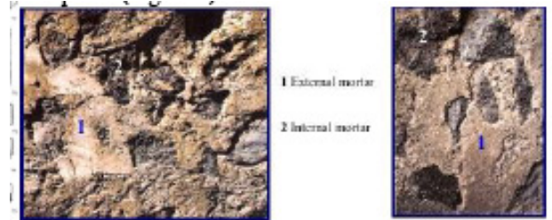
Fig. (9). External crushed mortar and internal mortar.
