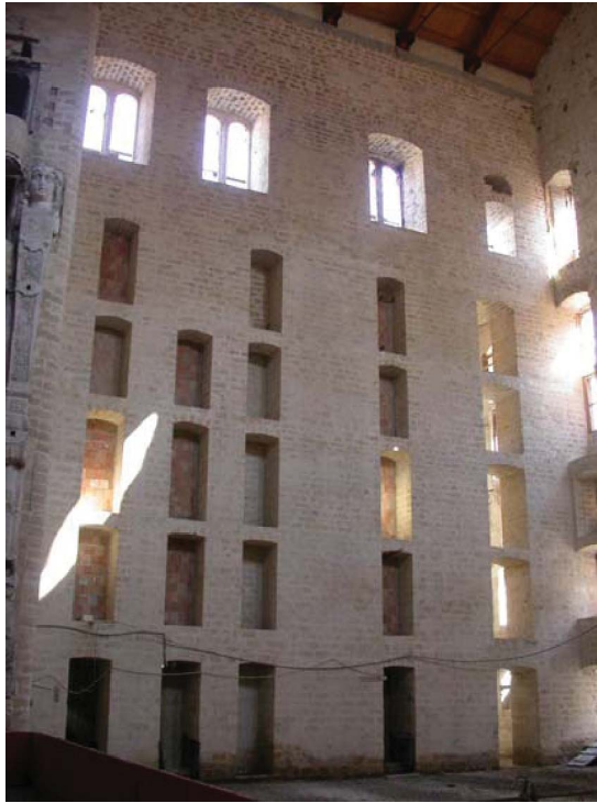
Figure 14. Photograph of the lateral wall of the fly tower and its frame model.
