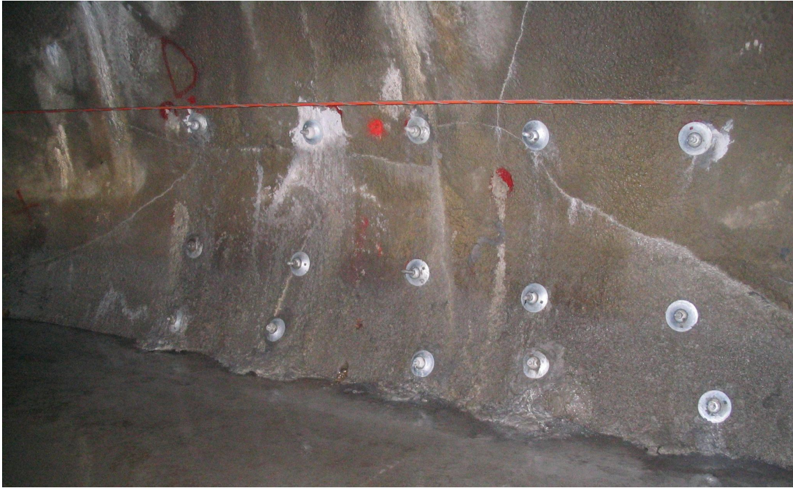
Fig. 5. Cracks in the shotcrete lining (design average thickness of 20 cm) of a water conveyance tunnel. The rock bolts were later installed to control and stabilize the lining. The cracks were induced by the presence of large irregularities of the tunnel boundary (photograph archive Prof. D. Peila).
