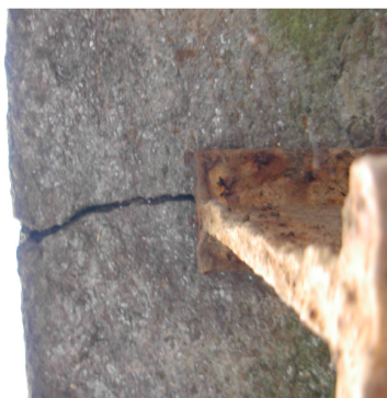
Figure 3: Details of a balcony where the beam leans in correspondence to a fracture.
