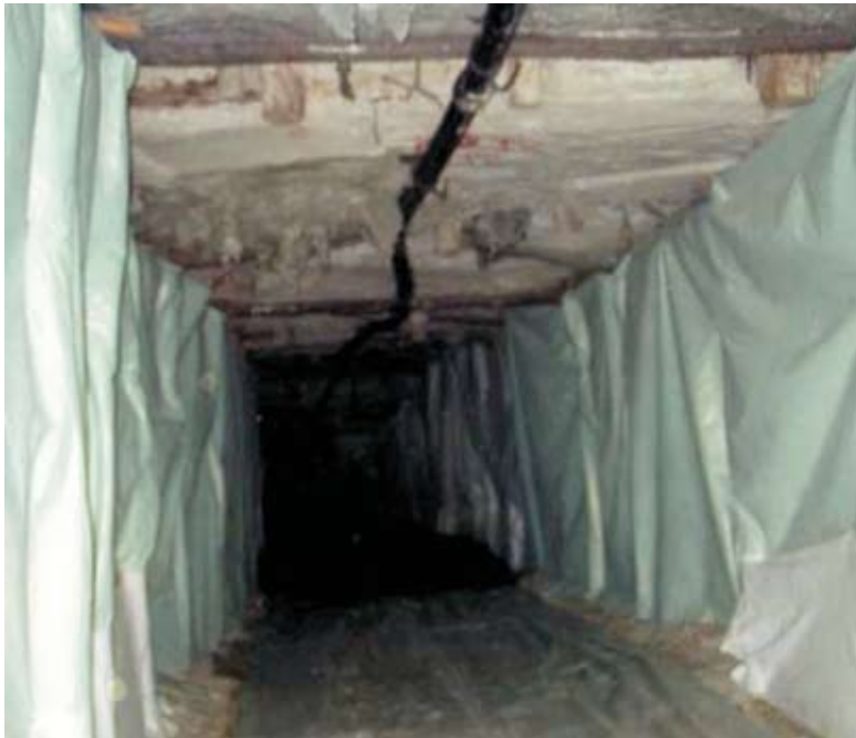
Figure 2. Scheme of the filling of a drift and photograph of a drift ready to be filled, where an impervious membrane has been installed to protect the not yet mined talc against pollution
