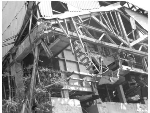
Figure 6. The state of building “B” showing the incipient risk for collapse.
