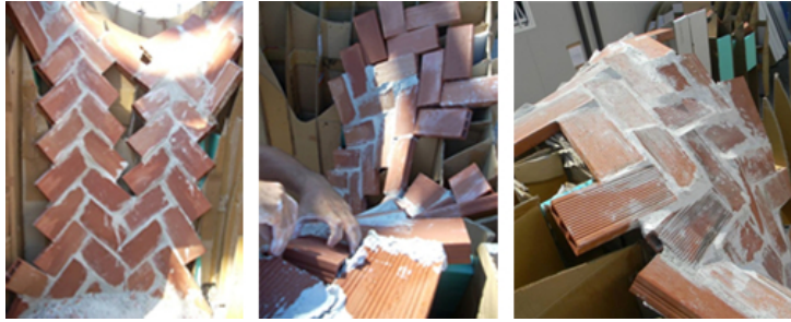
Figure 8.1: Brick laying problems in free-form vault construction
