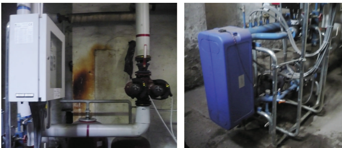
Fig. 2. Case study district heating sub-station.
