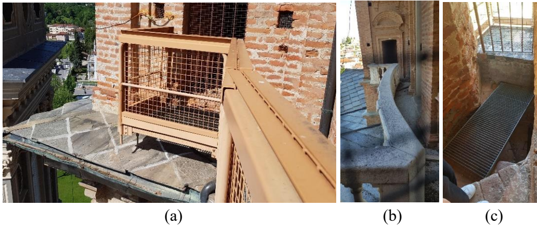
Figure 6. 10: external balconies in location 4: metal (South side) (a) and masonry (West side) (b). Dangerous access to the West balcony (c)
