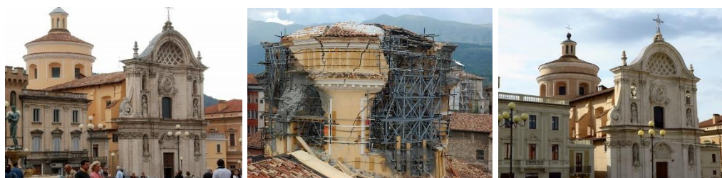
Figure 1. 2: pre , during and post phases on the Anime Sante church (L'Aquila, Italy) damaged by the 2009 earthquake
