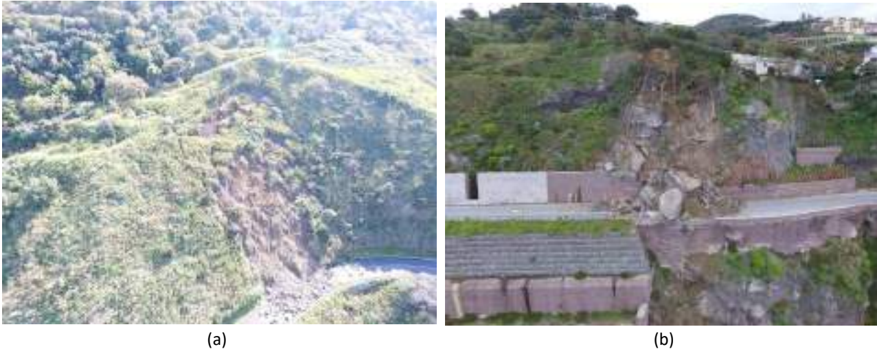
Figure 1 - Landslides events occurred in the municipality of Gioiosa Marea (ME) in March 2016): a) a debris flow on SS113 km 87+060, and b) a rockfall on SS113 km 87+600.
