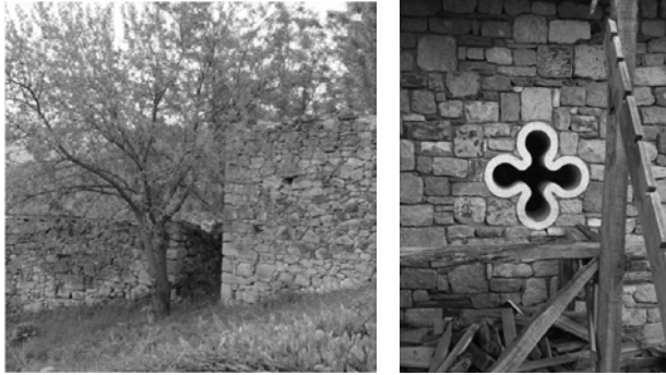
Fig. 7: Material displacement/replacement: stones from the old village houses in the church wall.
