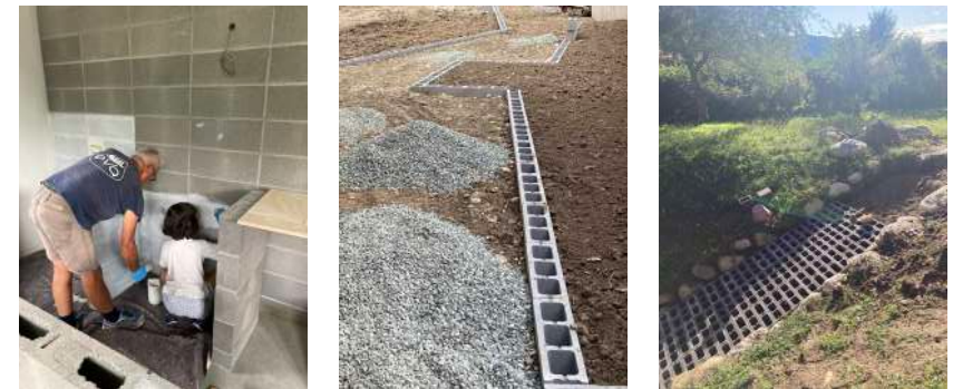
Casa BM, The ductility of the concrete blocks. Cladding the living area. Dividing walls across both floors. Garden borders. Paving to manage surface water on the slope down to the basement. Leftover blocks of different thicknesses, which would otherwise have been discarded due to the small quantity of remaining material, were reused to build the kitchen walls, whose design is defined by the sequence of partitions with varying thicknesses. Photo: ErranteArchitettura
