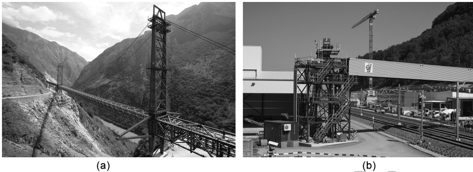
Figure 6.5 Belt conveyor over a gorge (a). Belt conveyor crossing railways and streets (b). (Courtesy of Marti Technik.)
