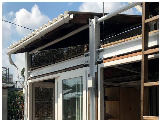
Figure 10 | Mobile system roof and flexible water recollection solution. Source: PEI Team.
