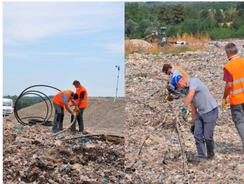
Figure 5. Phases of preparation and installation of the electrodes for borehole and cross-hole monitoring of electrical resistivity. The graphite electrodes are installed on the external side of the HDPE tube of the piezometers.
