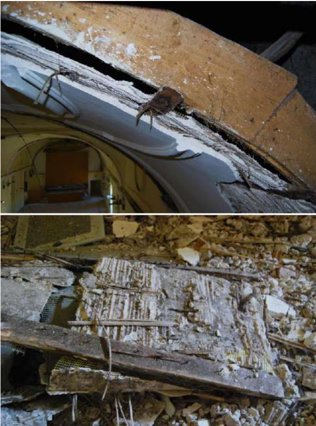
Fig. 5: Photographies of the damaged vault extrados details. (Post-earthquake 2009)
