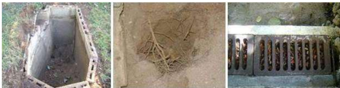
Figure 5. Evidence of technical and maintenance deficiencies in the infiltration works.
