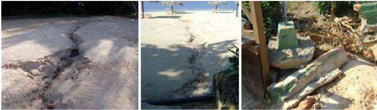
Figure 3. Sample of hydric erosion evidence in the berm, and green areas adjacent to strata 1 and 2.
