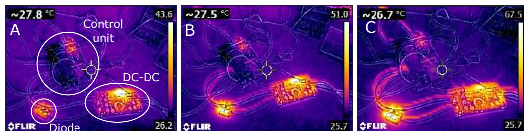
Figure 9. Images collected during the thermal test with the thermal camera: (A–C) correspond respectively to 100, 200 and 300 W of power flow.
