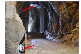
Air direction and speed monitoring.
