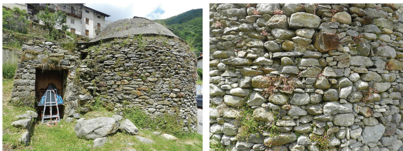
FIGURE 7 The Ice-House in Piedicavallo (left); A Detail of the Stone Masonry (right)
