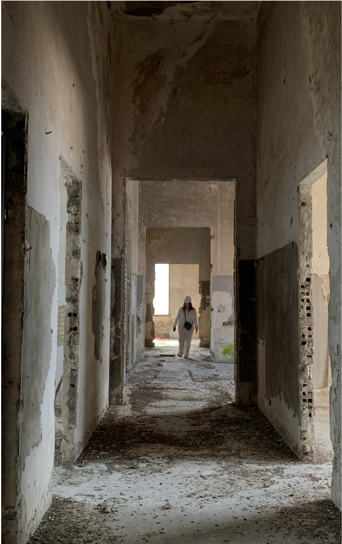
Site survey to Former House of the Fascist Party, Predappio, Italy, June 2025
