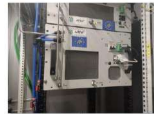
Figure 2 Installed electrolyser at ZEM module
