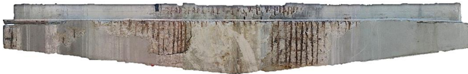
Figure 13: Effects of steel corrosion on pier cap.
