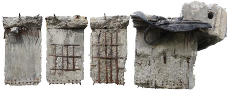
Figure 14: Corrosion scenario at the end of the girders adjacent to pier cap 46.
