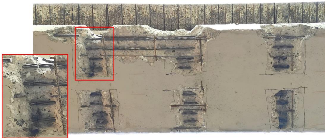
Figure 23: Strands cutting in B5-P47/46 girder (bottom view).
