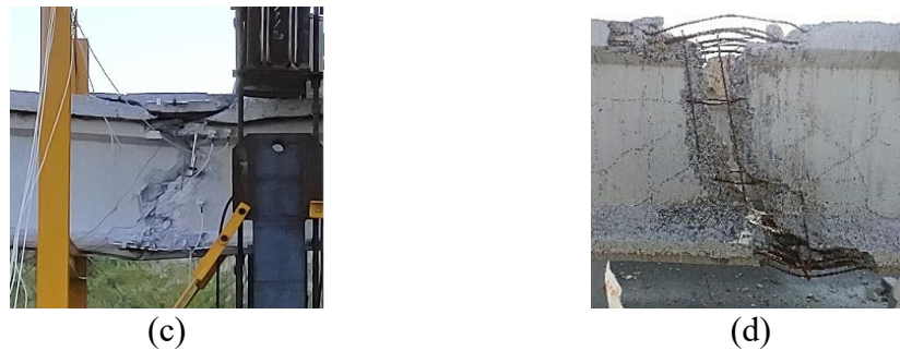
Figure 28: Detail of the failure zone: (a) B3-P47/46, (b) B8-P47/46, (c) B4-P47/46, (d) B9-P47/46 girder.
