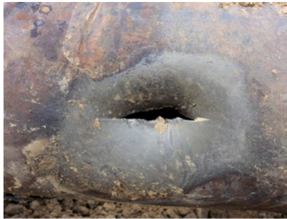
Fig. 2. Typical excavator puncture on pipe surface.
