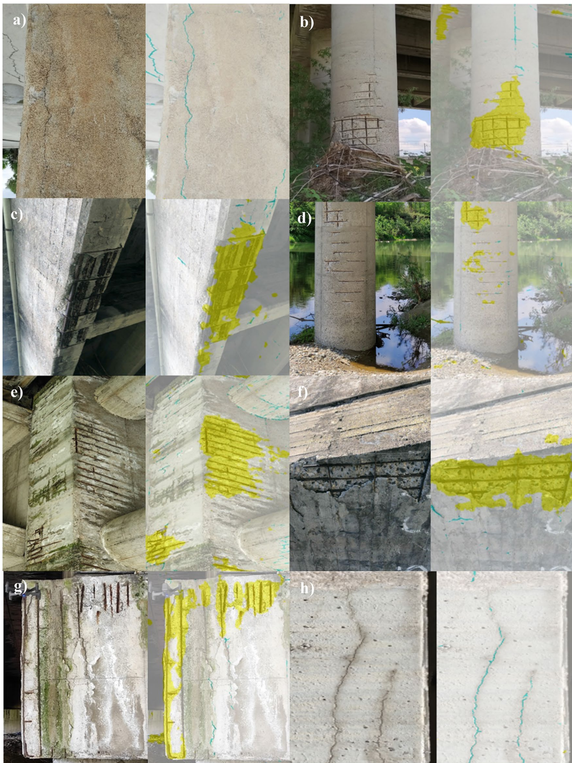
Fig. 11 Test images with high-resolution: a underside of stairs; b piers; c girders; d piers; e pier cap; f abutment; g pier cap; h concrete surface
