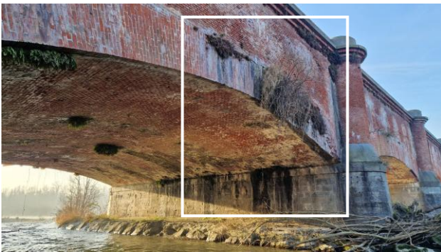
Figure 2. Example of water infiltration and vegetation undermining the structure.
