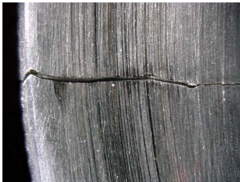
Figure 9. Crack in the FS rim.
