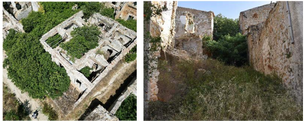
Figure 9. Presence of trees and weedy ground vegetation compromising, in some cases, masonry structures themselves (authors’ photos).
