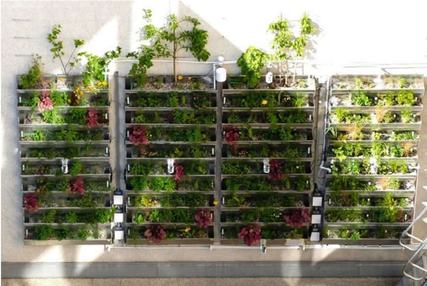
Fig. 28.3 Vertical greening system at the University of Natural Resources and Life Sciences Vienna (BOKU), Vienna, Austria. The system has a total size of 6m x 4m and consists of four individual systems with their own irrigation system. Monitoring included air and substrate temperature, substrate water content, precipitation, solar radiation, irrigation water volume and system output [13]
