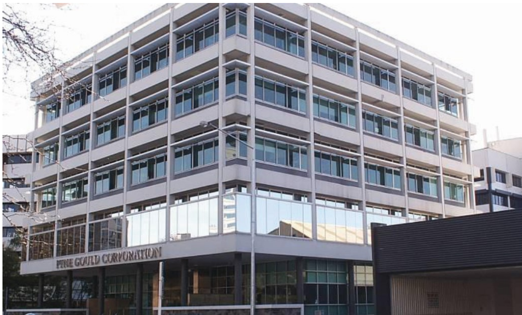
Figure 41. Pyne Gould Building photographed from the South-East elevation after the 4 September 2011 earthquake.
