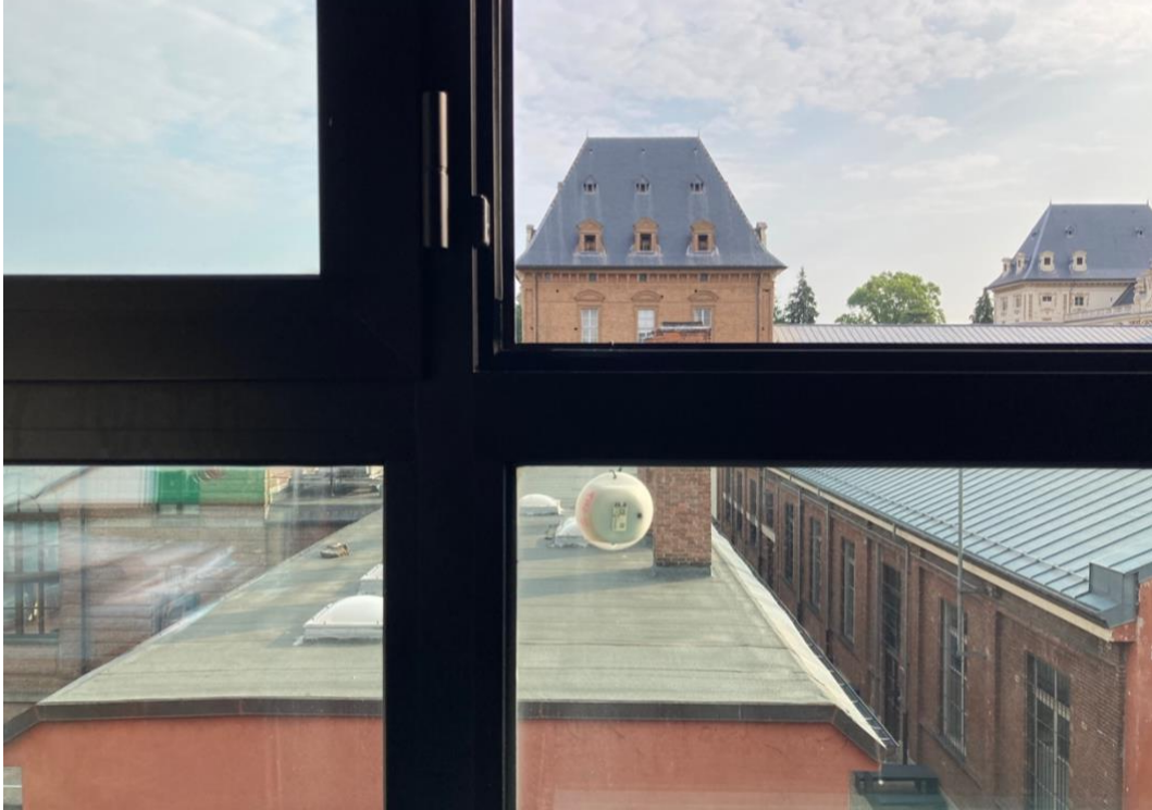
Figure 46: RFID sensor installed on the external façade during the Test B
