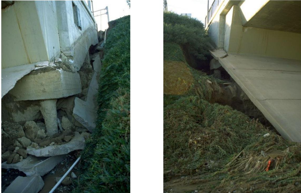
Figure 2.5. Typical abutment damages during the Northridge 1994 earthquake [36].
