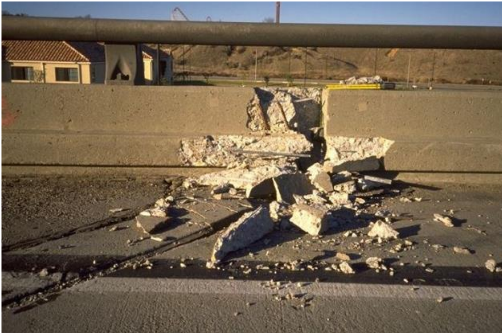
Figure 2.3. Local damage at the expansion joint during the Northridge 1994 earthquake [36].
