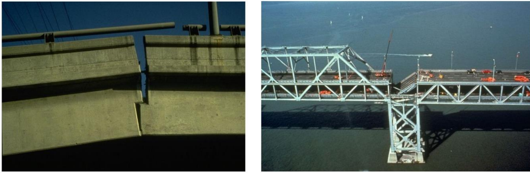
Figure 2.2. Typical superstructure unseating during the Northridge 1994 and Loma Prieta 1989 earthquakes [36].
