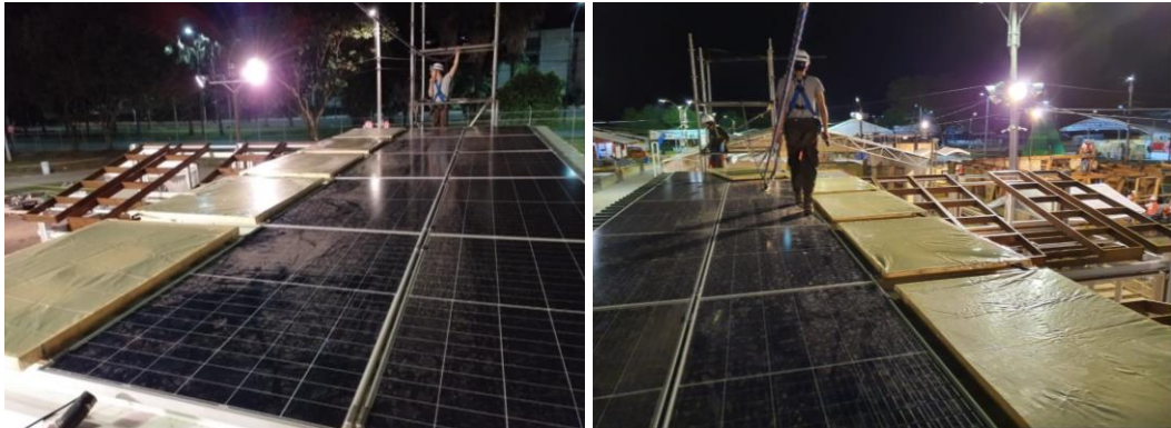
Figure 117. Positioning of the solar collectors on the roof next to the photovoltaic panels. Source: PEI team, 2019.
