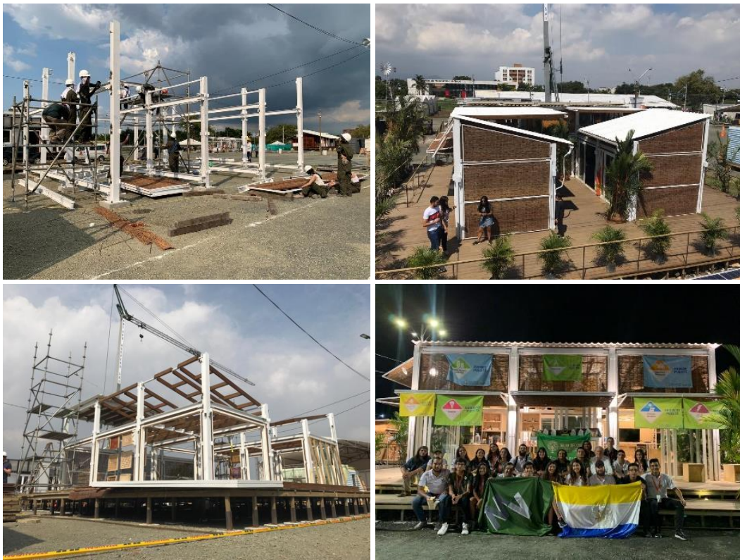
Figure 101. Photos of the PEI Máquina Verde-El Arca housing prototype during and after construction at SDLA&C 2019.
