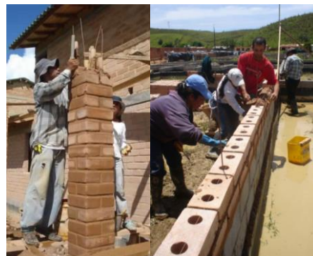
Casa Viva neighborhood (compressed stabilized earth block) / Fundación Tierra Viva. Vegachí, Antioquia (CO).
