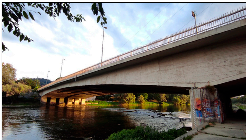
Figure 8. Close-up view of the Corso Regina Margherita Bridge (V1-T), which is the subject of this and other ongoing research.
